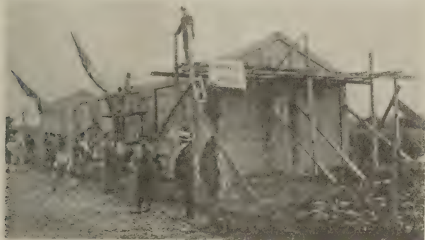
This photograph shows the masonry work completed for the first building in one of the villages of the Mugello district, wrecked by earthquake
